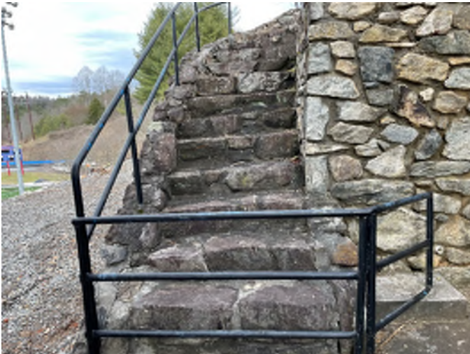
^ Pipe rails to be removed, build up first few steps with salvaged rock to create stone planter
